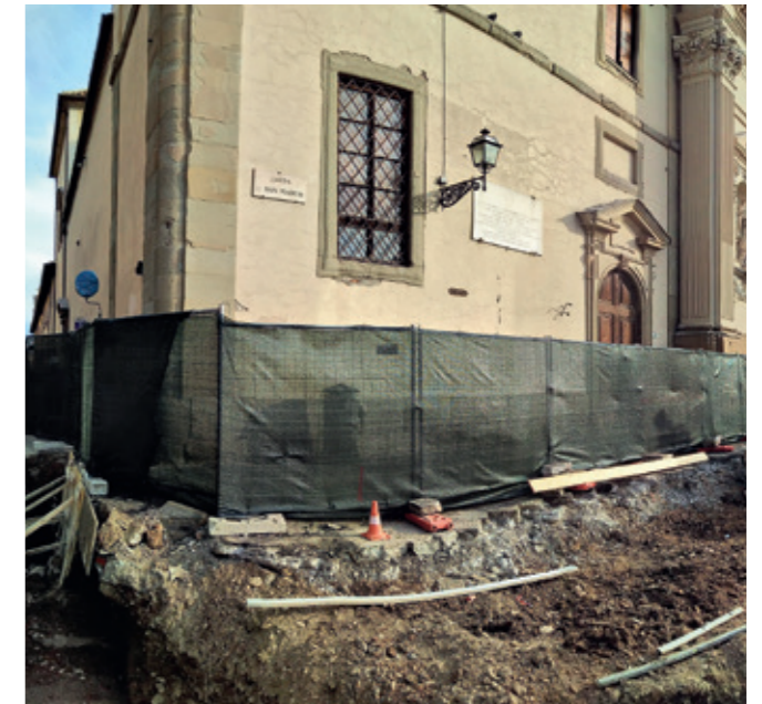
Ante operam works: excavation for the insertion of NoViDamp anti-vibration panels to protect against vibrations produced by the transit of trams, buses and heavy vehicles in the Basilica of San Marco in Florence
